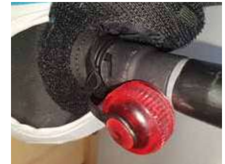
Photo 19: Hose with coupling attached to valve.
